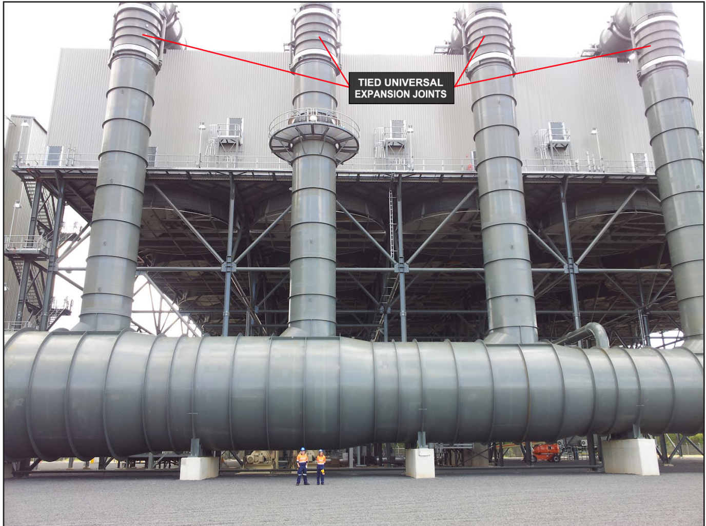
Figure 6 Exhaust Riser Tied Universal Expansion Joints
